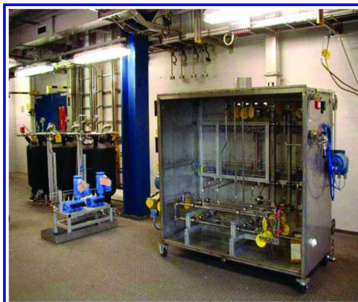
Figure 17. Pilot plant DFT unit
